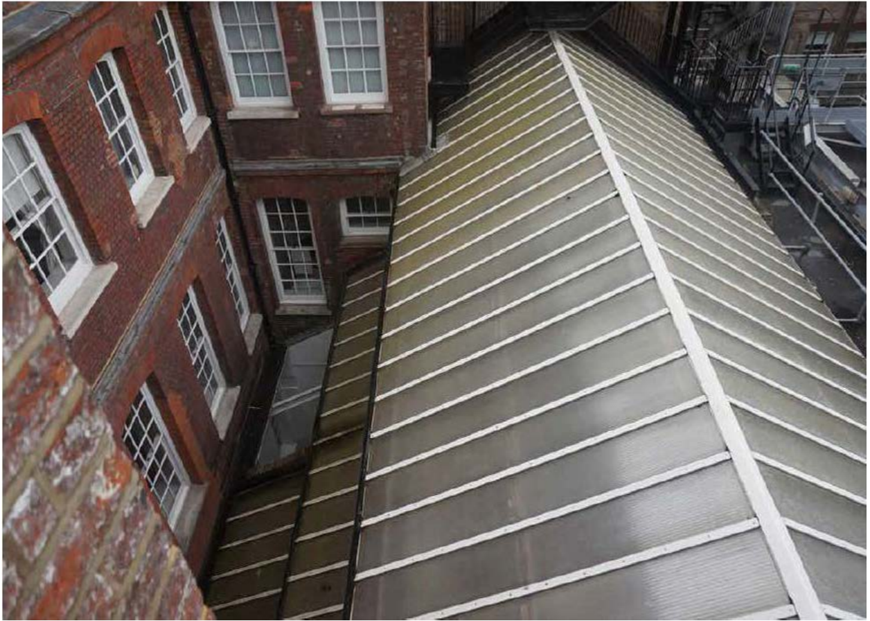
Atrium roof of 11 Floral Street adjacent to 43 King Street (Prior to works to refurbish atrium glazing)
